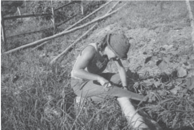
HRDC Intern Sarah Weinberg constructing a staircase for the local marketplace in Manglaralto, Ecuador
